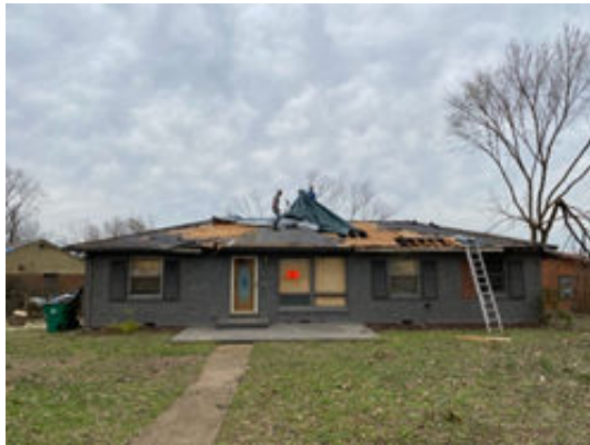
Property after tornado
